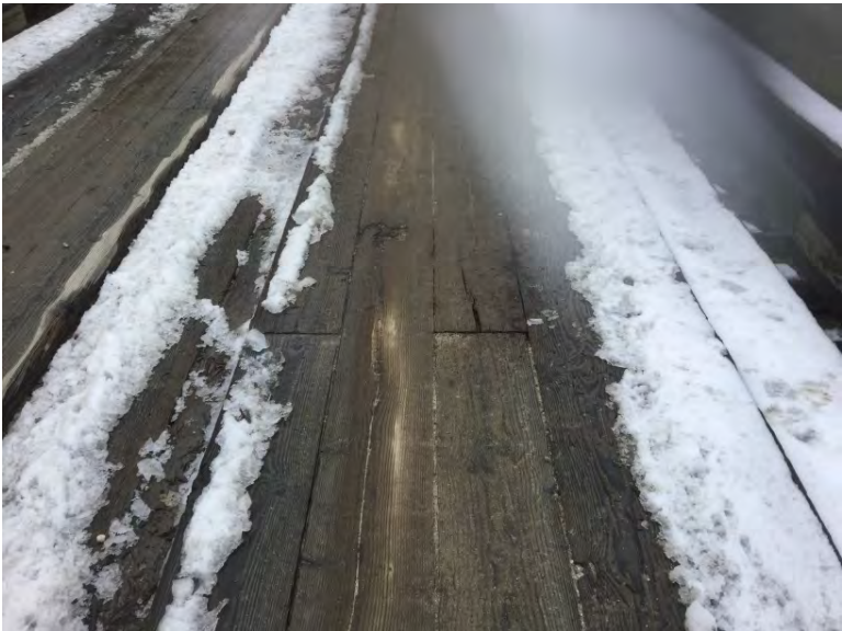
Minor wear on wheel path planks
