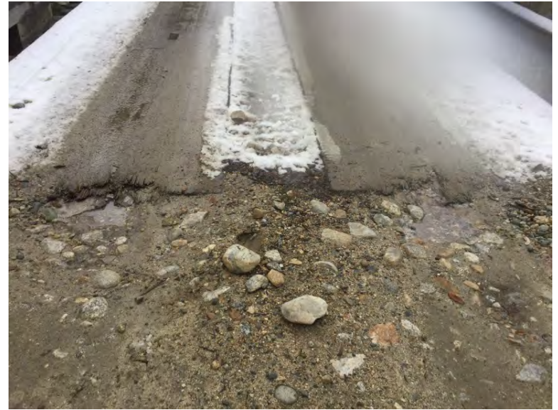
Minor wearing of planks at each approach
